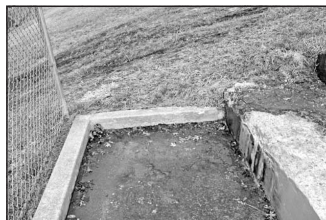
Photo by Shawn Jarrard Groundwater has made the TCHS baseball field unplayable and has worked its way down to the concrete bleachers in Frank McClure Memorial Stadium.
